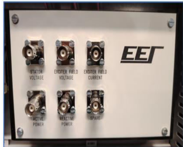
(Figure 2 - BNC Test Panel)
